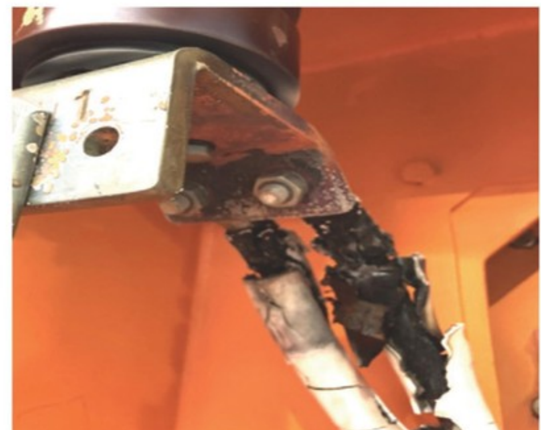
8. Failing motor tail connection
