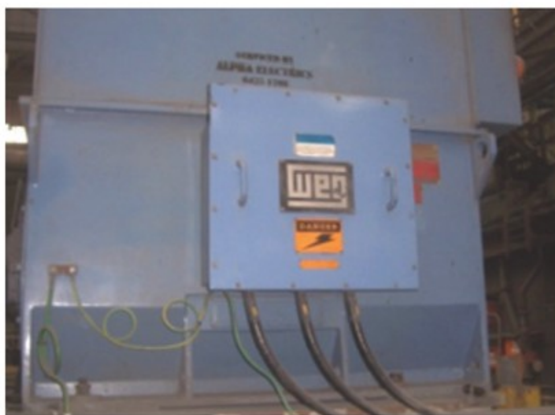
5. Junction box with cover in place
