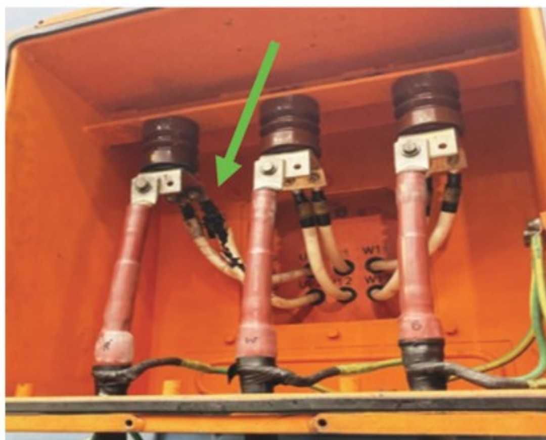
7. Cover removed showing three phases
